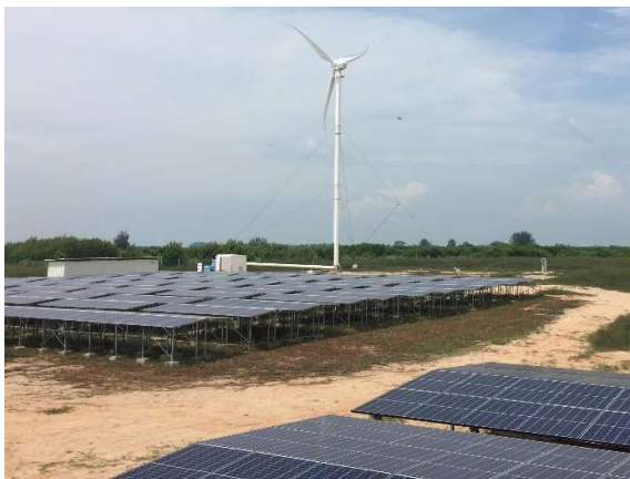
Figure 1: Wind turbine & PV panels in Semakau Island
